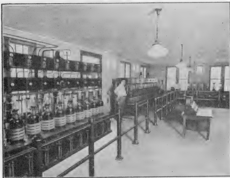
FIG. 322c.—A general view of the 32 water-cooled tubes with which the WEAFF transmitter at Bellmore, Long Island, N. Y., is equipped. The water circulates through the coils of rubber hose at the base of each tube. Each tube is equipped with a relay which drops and displays a small white disk in the case of tube trouble.
