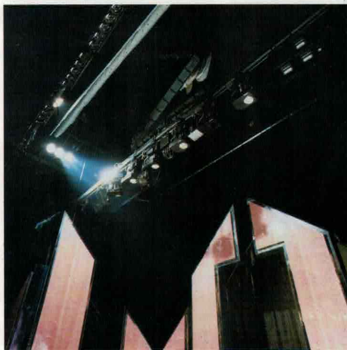
12 PEF-M motorised lighting units were installed at the Volkstheater, Vienna by Ludwig Pani in 1980.
