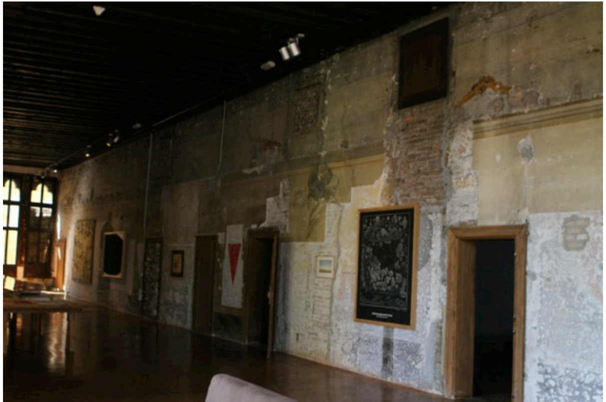
Fig. 21 Traces of the half-floor along the upper part of the wall on the second floor of Palazzo Fortuny. Photo Zeke Smith.
