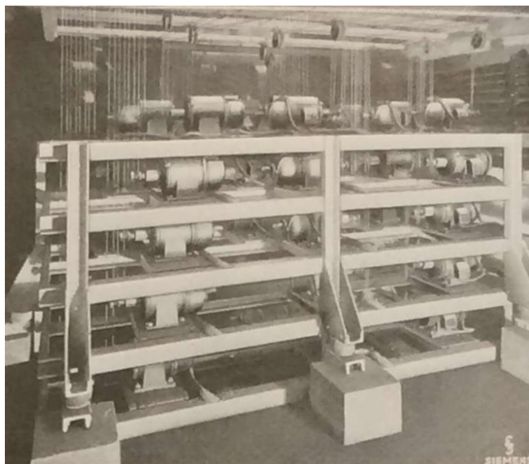
Figure 48. 60 Colour filter and mechanical dimming selsyn sender motors (Gerbermotoren) at Paris Opera, 1937. (Mosebach 1937)
