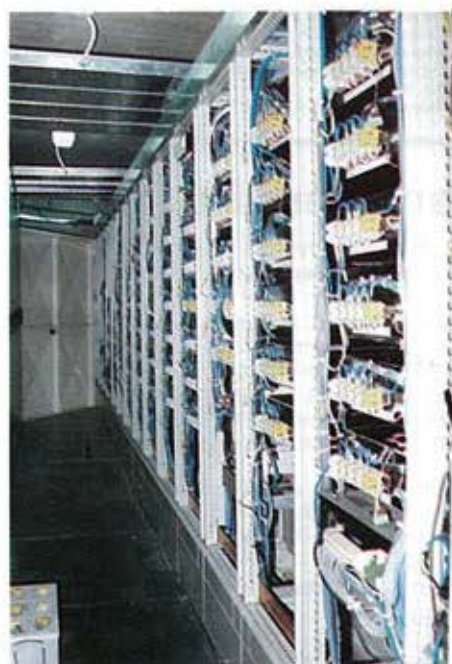
The Winter disco central dimmer room.
